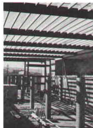
Expansion of Stanford Plant's Building 1 will allow growing space. Solid State group will move into new area early in 1967.
