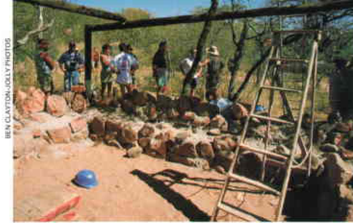
The HP participants had a chance to see firsthand the kind of construction work that Raleigh teams undertake during a visit to a remote location in the Waterberg Plateau Park.
