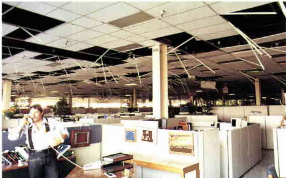
Ceiling tiles fell in many HP buildings during the quake. During cleanup at the Sunnyvale site, Jack Gephardt of facilities uses the phone of GM Bob Puette to make a report.
