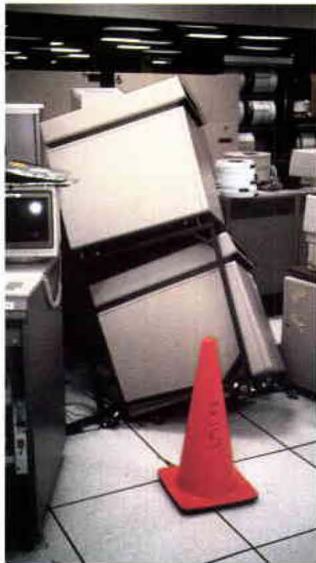
In Cupertino, seismic force slid this disk-drive rack into a floor opening.
